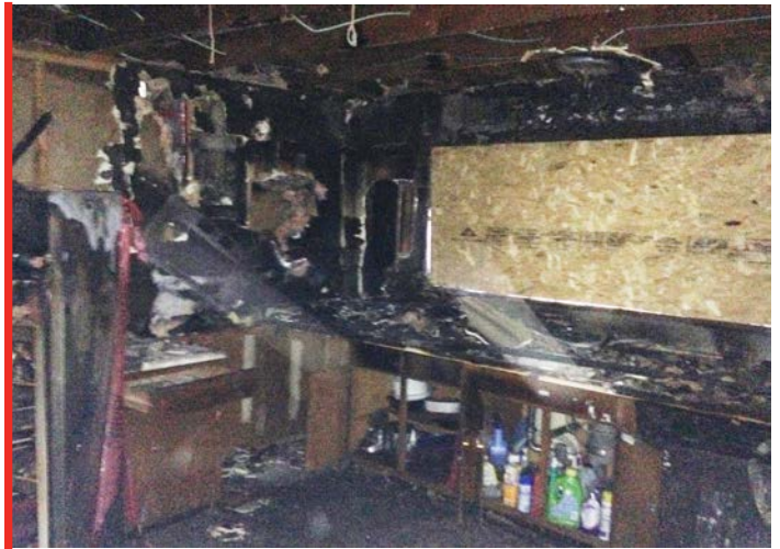
PHOTO OF FIRE DAMAGE AT REYNOLDS RESIDENCE -PHOTO COURTESY OF DAVE WILSON
